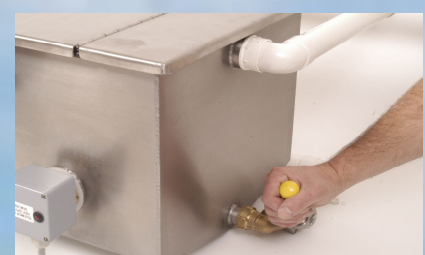
Open Silt Valve 5 Seconds - Daily
